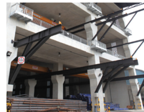
Loading and unloading facilities
